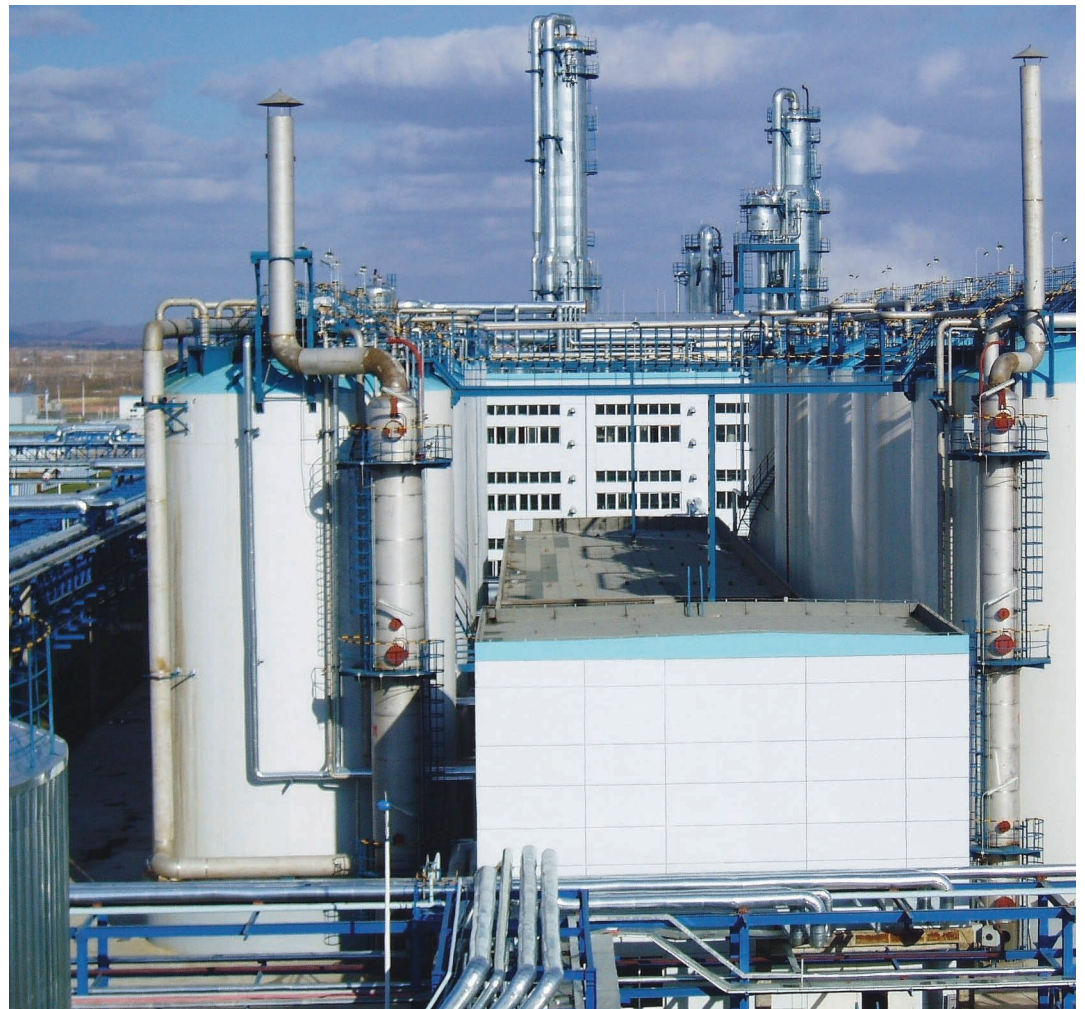
With a capacity of 1.25 million litres per day the distillery of Jilin Fuel Ethanol is Asia's largest bioethanol plant and at the same time the largest multi-pressure distillation system realised by Vogelbusch
